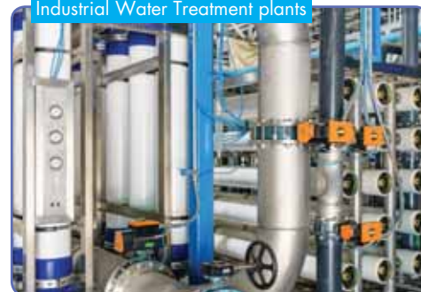
Industrial Water Treatment plants
